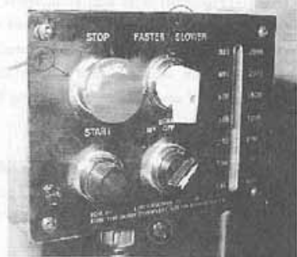
Figure 5 - Speed Control box
